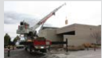
It took aerial acrobatics to hoist an 800-pound cold water coil for an air handling unit to the roof of the Joe Dini Library & Student Center on the Carson City campus.
